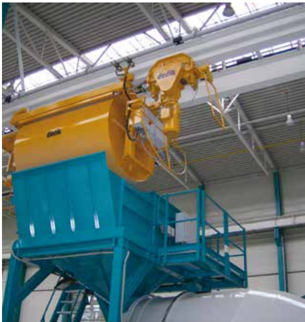
Discharge into the distributor
