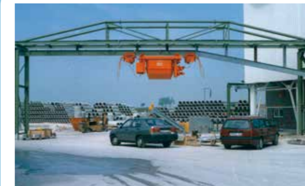
Rollover bucket in a bridge 25 m
