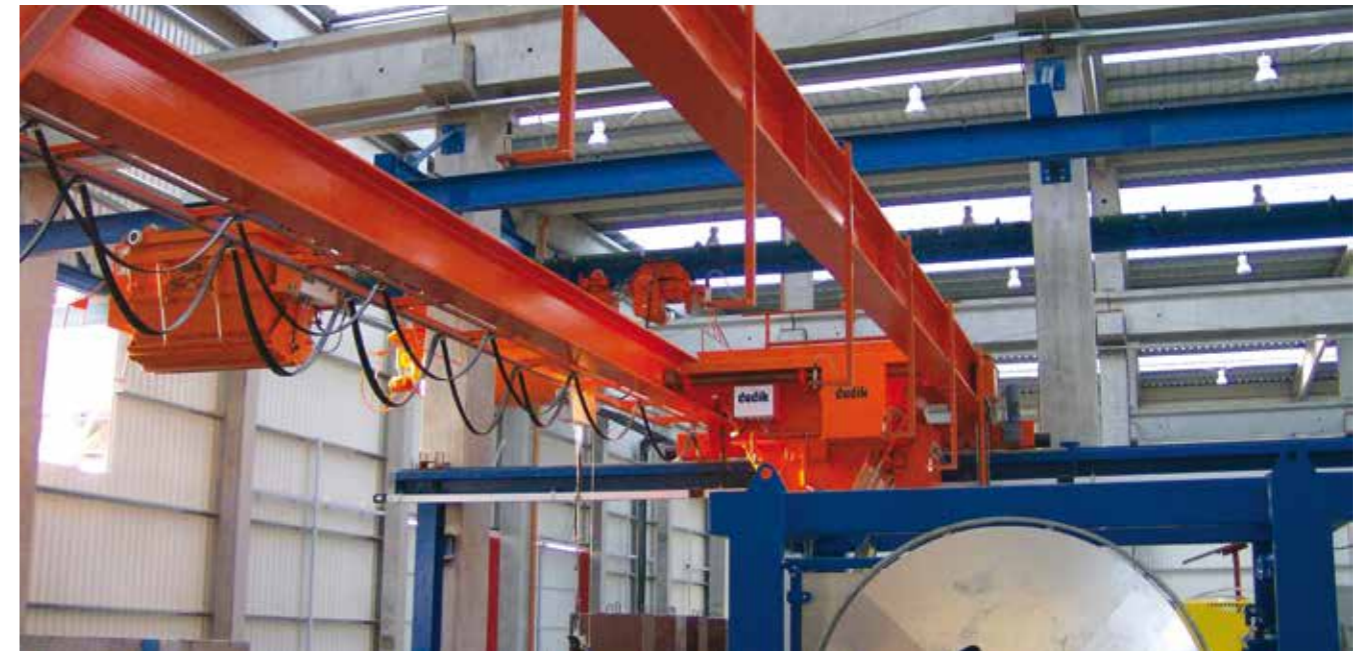
Automatic return travel of the skip conveyor to the concrete distributor, and from the concrete distributor to the extruder
